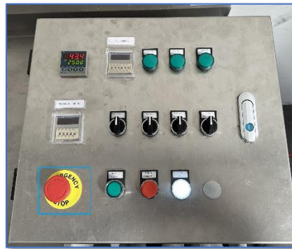
Figure 30 – PID Control Panel with Emergency Stop Button in Lower Right-Hand Corner Highlighted
