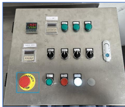
Figure 30 – PID Control Panel with Emergency Stop Button in Lower Right-Hand Corner Highlighted
