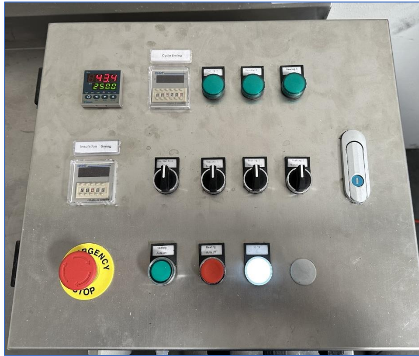
Figure 2 – PID Control Panel
